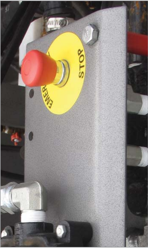
Emergency Shut Off Switch ("Panic Button")
