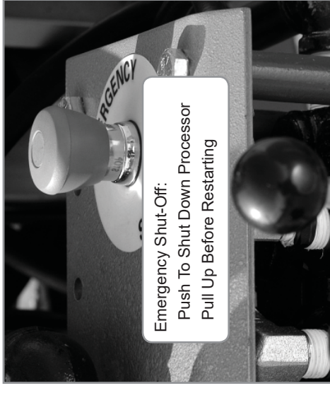
Power Plant Controls – Emergency Shut Off
